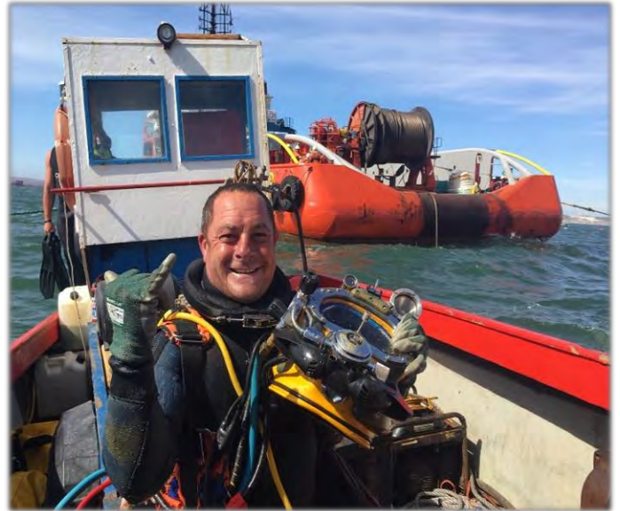
Connecting cables and shackles for Gas Pipe Saldanha
