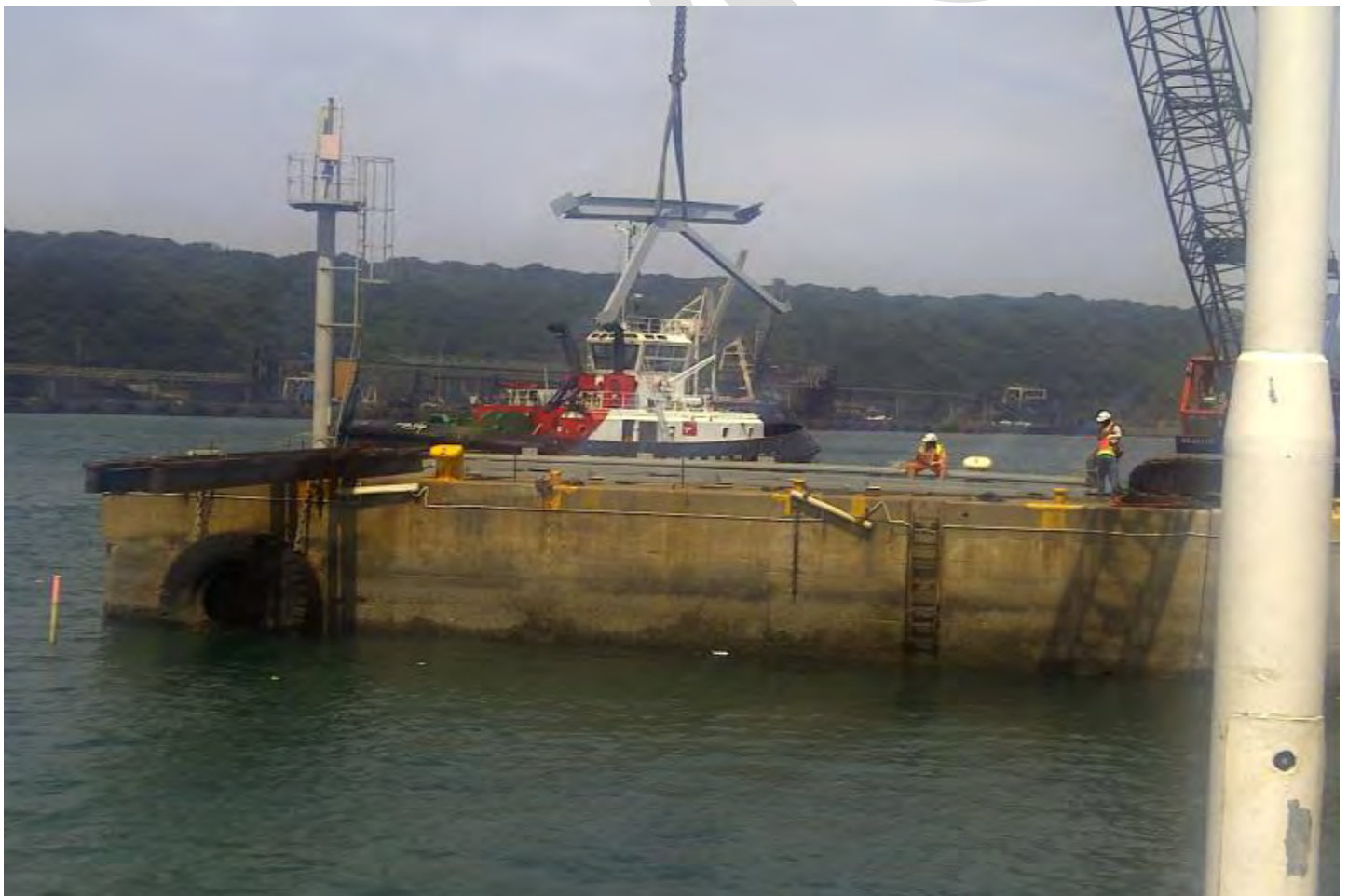
Dismanteling and Reconstruction of NSRI Launching Facility, Slipway System and Winche 2013 NSRI – DURBAN
